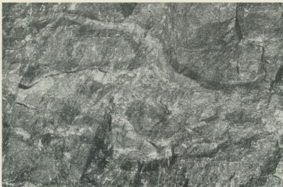
Fig. 7. Pyroxene-epidote skarn veins (appear lighter than the surroundings) brecciating cordierite-quartzite. Dark, hornblende-rich reaction zone with the quartzite. In the centre, a small inclusion of quartzite with a reaction zone. Roof of a tunnel, 165 m.-level, Adak Mine; 1 : 10.
