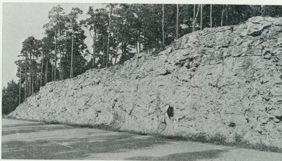
Fig. 1. Bofride 1. Photograph of the reference point, with an arrow showing the reference level.
