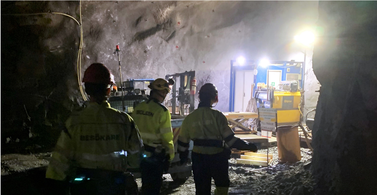
Drilling in the Kankberg Mine where gold and tellurium are the economically interesting substances. Photo: Carolina Liljenstolpe/SGU.
