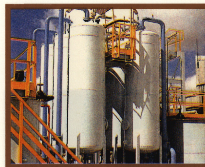
Carbon-filled steel columns for gold extraction at the Nalesbitan, Camarines Norte, mine of Goldfields Philippines Corp.
